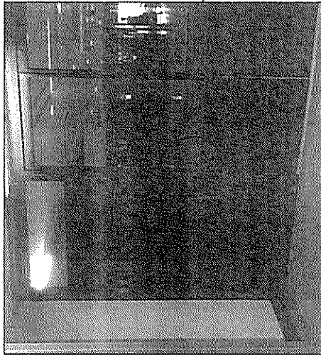
GLASS DOOR AT NORTH WING HALLWAY LEADING TO SECRETARIAT LOBBY 32" x 31" x 1/4" THK (1pc)
